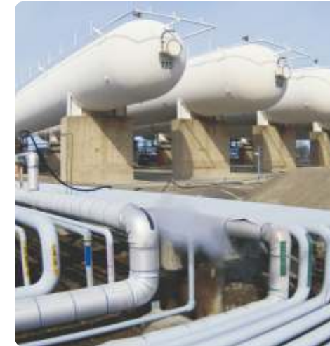
Onshore Oil & Gas Pipeline
